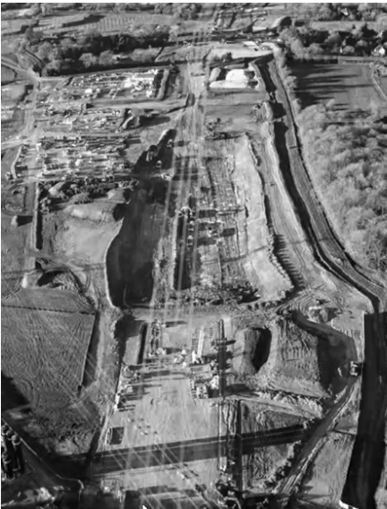
Excavations at South Heath, showing the start of the tunnel portal in the foreground
