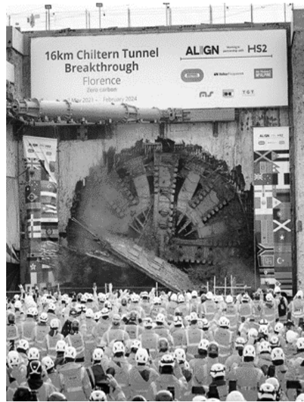
‘Florence’ - the first of the Chiltern tunnel TBMs - breaks through at South Heath
